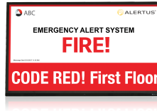
Digital Signage & Cable TV Override
